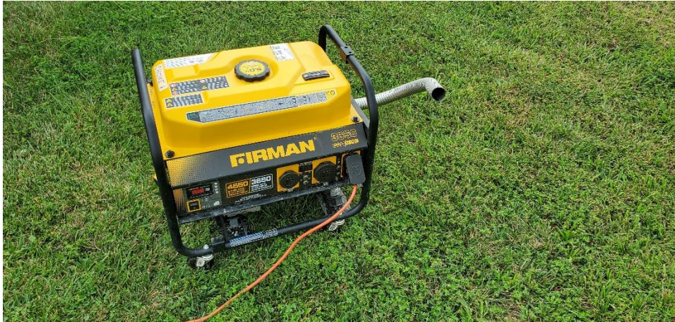
Generator used for 100% Emergency Power
