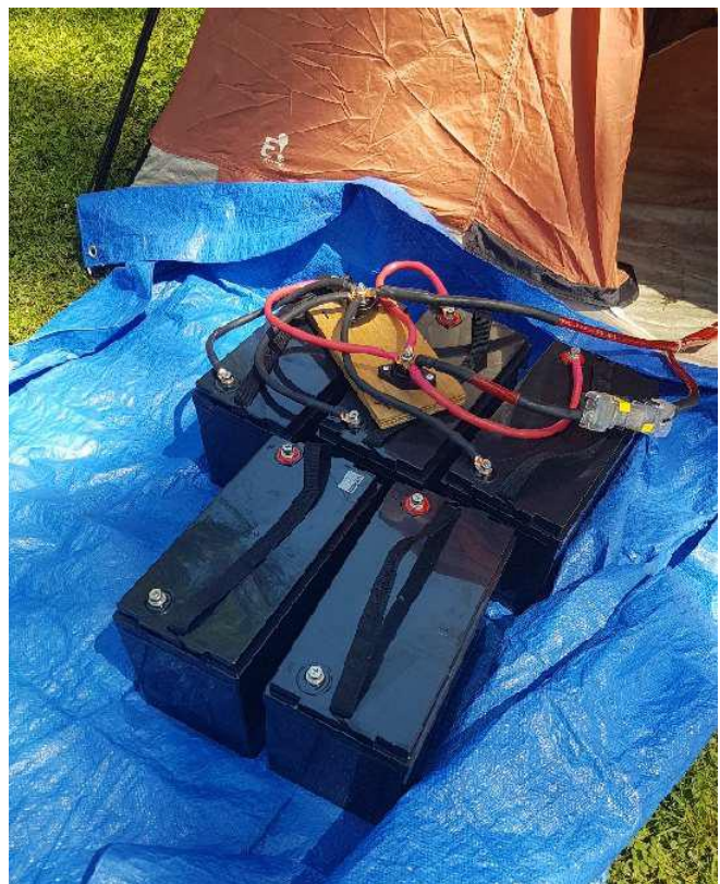
(5) LiFePO4 100 AHr Batteries for Main Power © VE2SI – Leo Nikkinen
