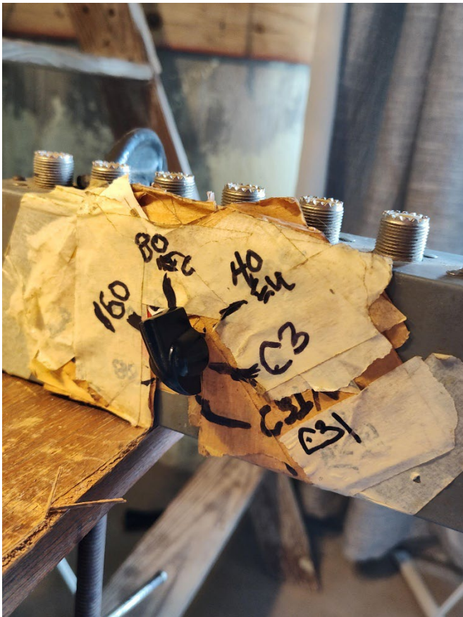
Salt water never stops. Parting ways after 35 years, W2GD discovered a coax switch at P44W that is beyond repair – photo courtesy of W2GD
