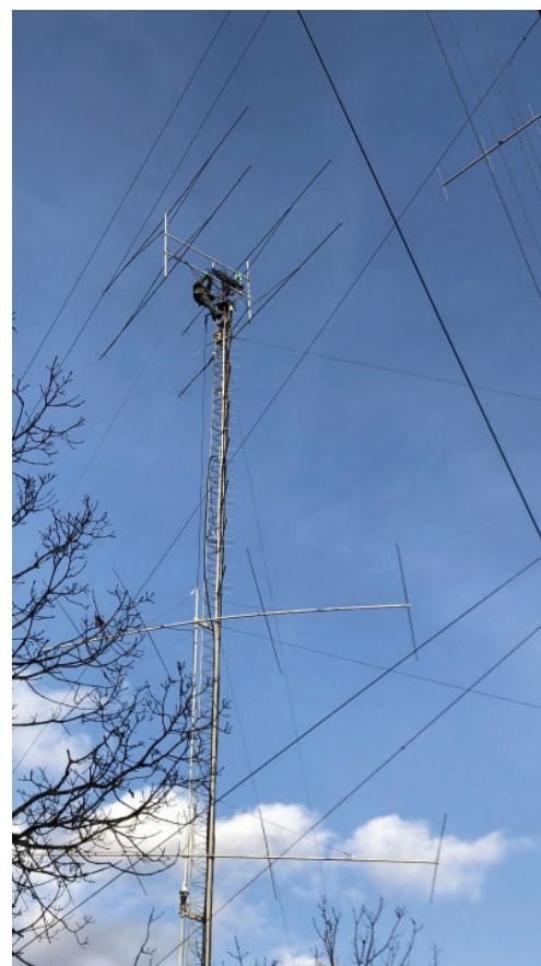
Dave Olean, K1WHS, performs pre-contest maintenance on his 222 MHz antenna array in preparation for the 2024 ARRL 222 MHz and Up Distance Contest. The antenna array consists of four 22-element antennas at 106 feet with azimuth and elevation rotation capability. [Dave Olean, K1WHS, photo]
