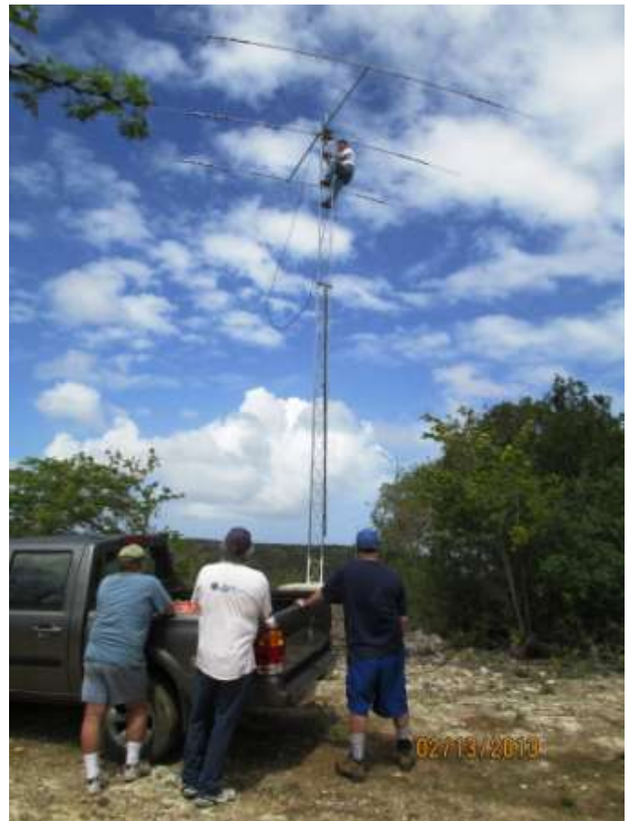
Installation before the contest of a receive-only tribander about one-quarter mile from PJ4X: Jeff, K1ZM is doing the heavy lifting on the tower. Supervising, supporting and encouraging from the ground were (L-R) Charlie, K1XX; Ken, K1EA, and Jim, W19WI. (PJ4X Team Photo)
